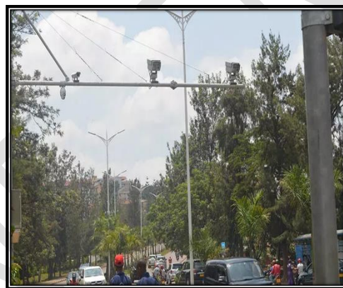
Figure 3: Road CCTV Camera Source: (aptantech, 2020)
